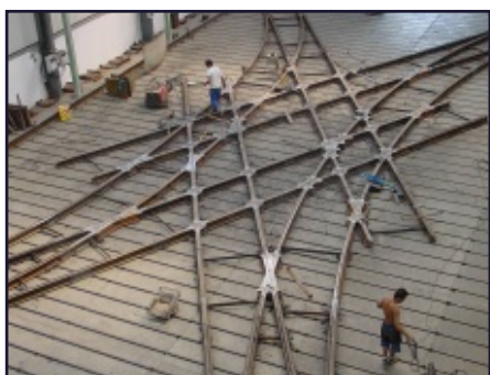
Rail crossing in the production hall
