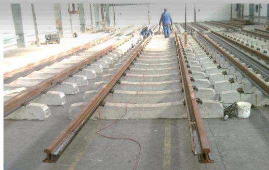
Grooved profile Spurrillenschiene 49E1 pre- assembled in Pražská strojirna a.s. on concrete sleepers and installed in Prague
